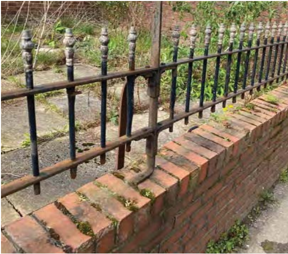
4.28 Historic and modern boundary walls, the latter with reused railings, and poor surface materials at Cornbrook Terrace
