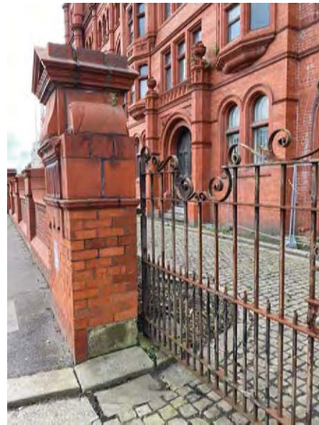
4.5 Ornate boundary wall and railings, with retained stone setts, at the Essence Factory
