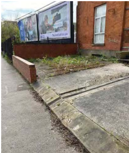
7.2 Loss of boundary wall and garden to Cornbrook Terrace
