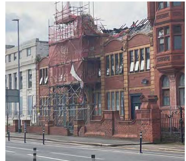
7.9 Deterioration at the Trafford Press building
