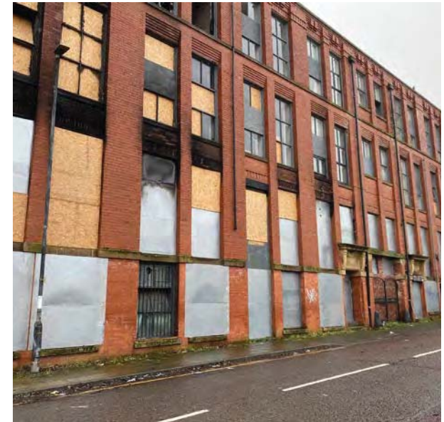
7.8 Fire damage to Empress Mill
